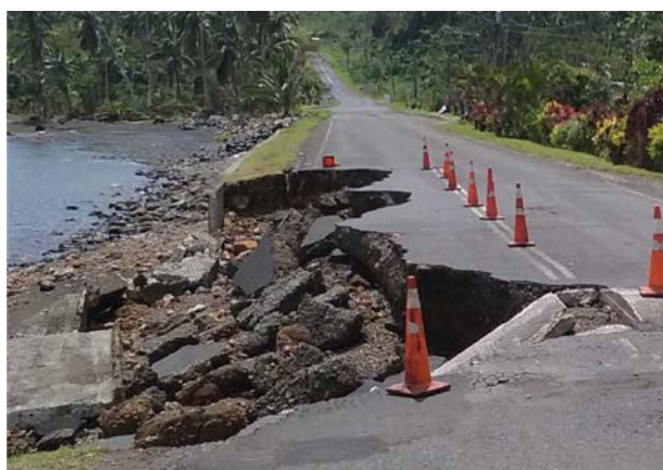
Figure 18: Damage to roadway after Cyclone Winston
